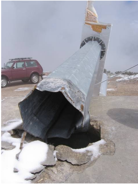
Figure 6. Column of wind genetaror after third intervention by a company that it was mounted.
