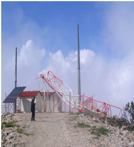
Figure 7. The instability of wind generator column.
