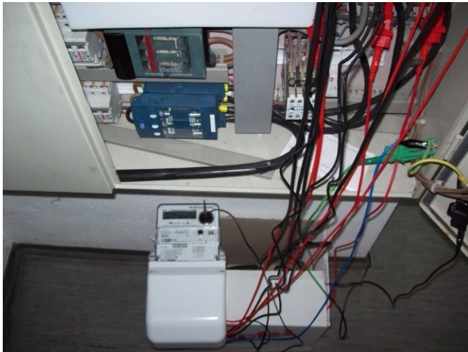
Figure 4. System in operational state on site.
